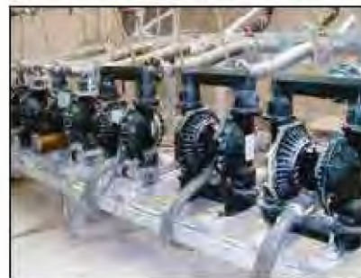
3" diaphragm pumps mounted on a skid to transfer clay in a ceramic manufacture
